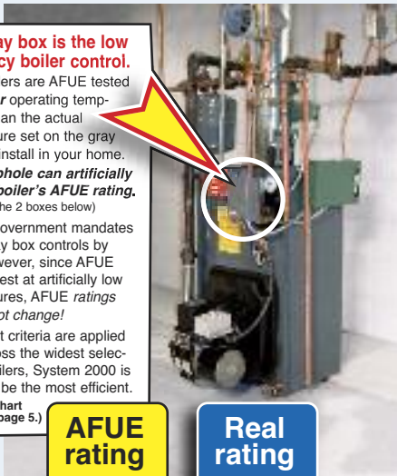
Cast iron tankless coil boiler.
