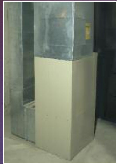
Hydro-air and heat pump backup
